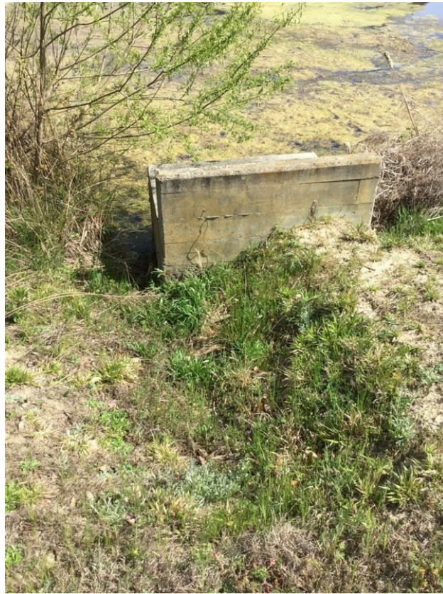
Erosion on sides of riser F12509- 1023
