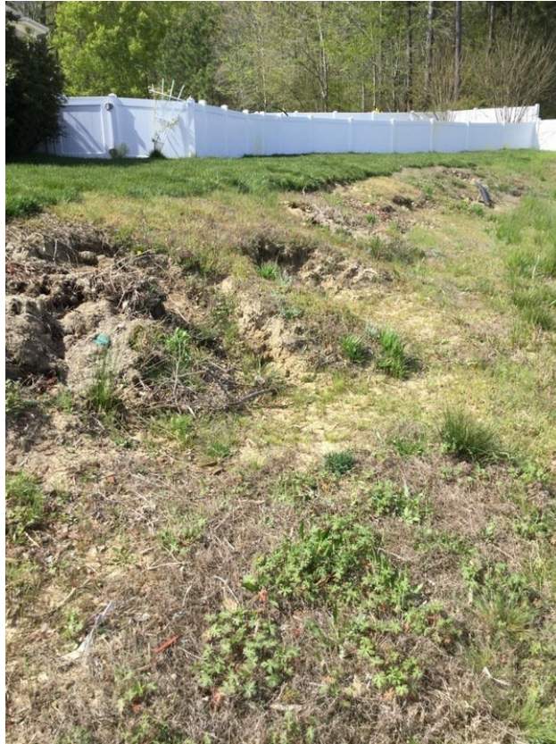
Large amount of erosion on side slope
