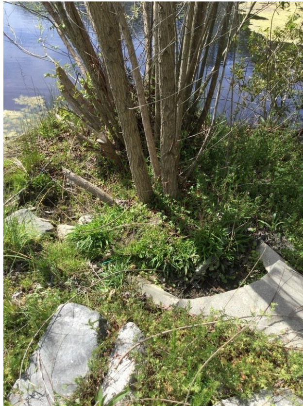
Overgrown vegetation blocking inlet
