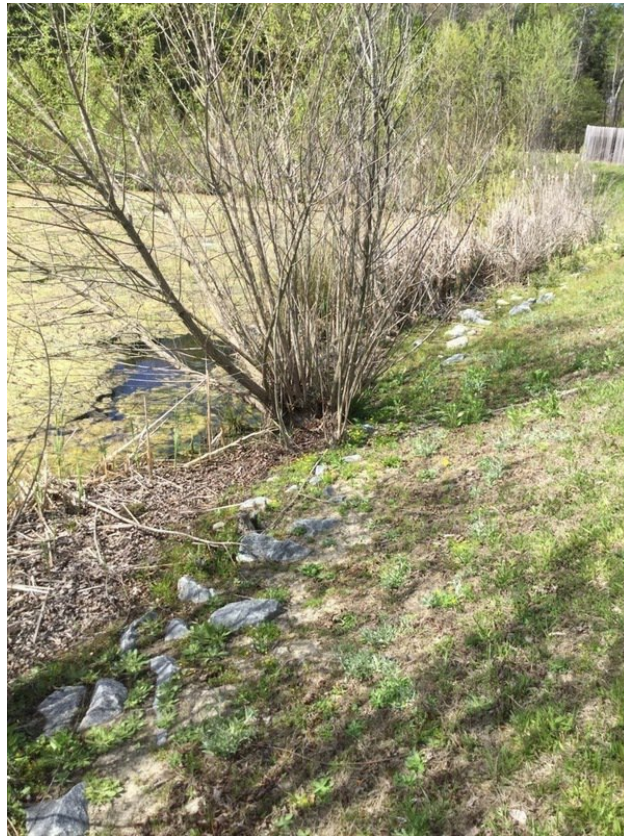
Some woody vegetation that may lead to future erosion
