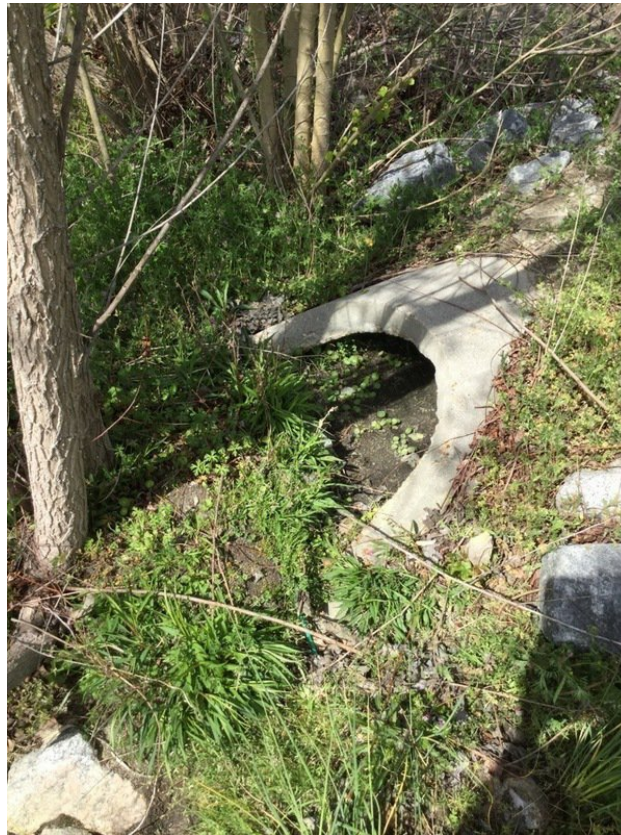
8" sediment deposit depth in pipe
