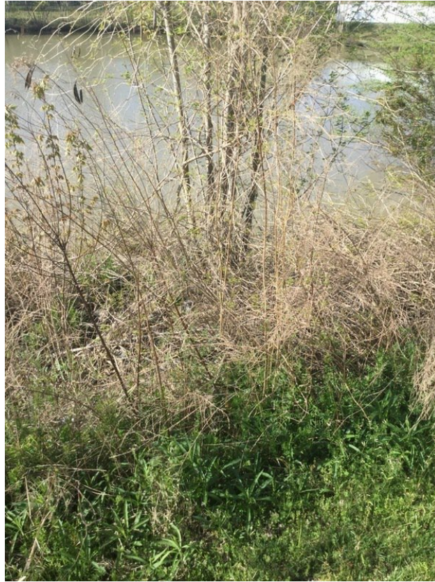
Woody vegetation overgrown around pipe. No other visible defects.
