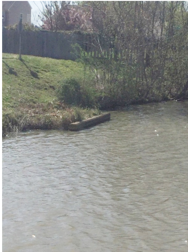
Structure submerged, but looks to be in good condition. Shown on map as a storm node.
